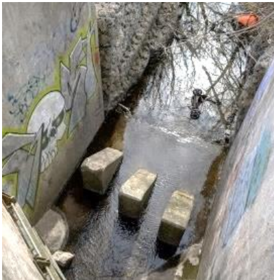
Stormwater enters Hungry Hollow ravine and Silver Creek via several outfalls. Erosion, sediment accumulation, scouring and corrosion, and increased litter and garbage are evident at outfalls. Photo Credit: CVC
