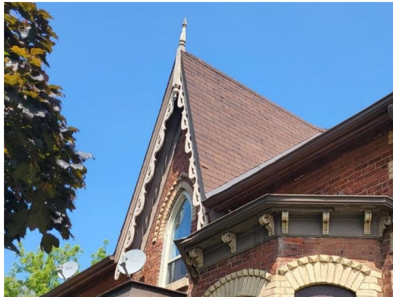
Figure 20: Detail of the central gable on the front (southwest) elevation of the existing building at 49-51 Main Street North, showing the decorative bargeboard and wooden finial (Town of Halton Hills 2025)
