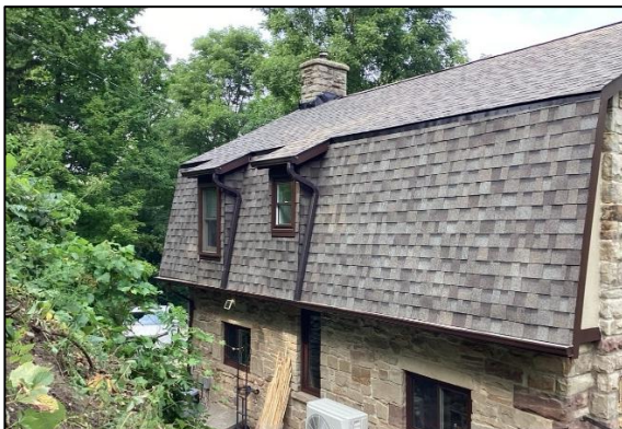
Figure 30: Rear view of the gambrel roof, showing two windows and new asphalt shingles (Courtesy of the Property Owner 2025)
