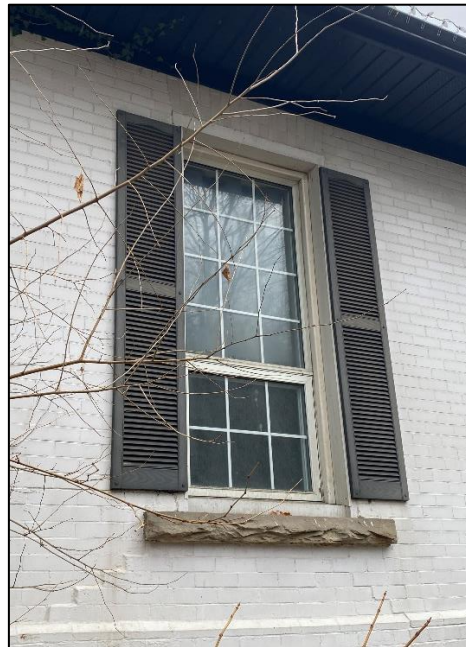
Figure 29: Original window along the side (northwest) elevation of the subject dwelling (Town of Halton Hills 2024)
