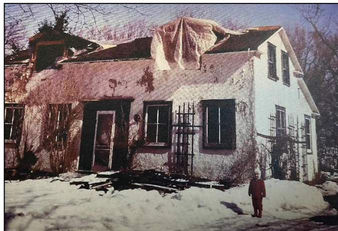
Figure 31: Extant dwelling under renovation in the late twentieth century, with new dormers above the roofline (Courtesy of Pamela Dickinson)
