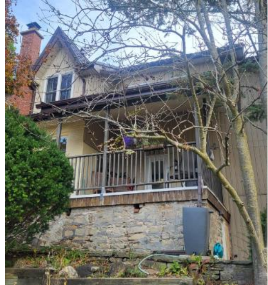
Figure 24: Side (southwest) elevation of the existing building at the subject property (Town of Halton Hills 2024)
