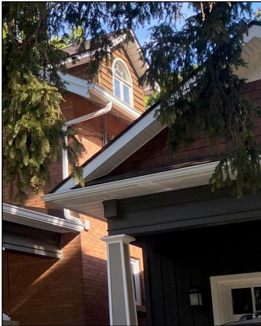
Figure 31: Partial side (southwest) elevation, showing the existing window opening and dormer (Town of Halton Hills 2023)
