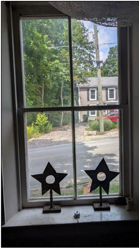
Figure 30: Interior windows along the front (north) elevation of the extant dwelling, looking towards Prince Street (John Mark Rowe 2024)
