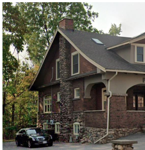
Figure 19: Northeast elevation of The Birches at 75 Mill Street (Town of Halton Hills 2023)
