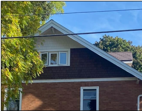
Figure 27: Existing cedar shingles beneath the gable peak, along the front elevation (Town of Halton Hills 2023)
