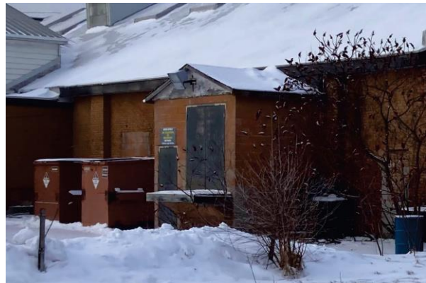
Figure 32: Detail of the cinderblock addition at the north end of the east elevation (Metrolinx 2022)
