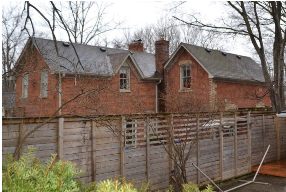
Figure 27: Rear elevation of the existing building at 14-16 Queen Street (Town of Halton Hills Files, 2018)
