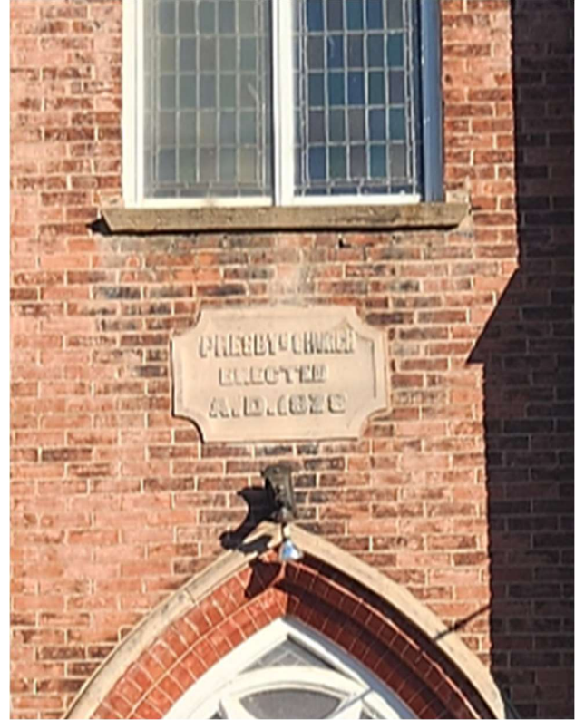
Figure 33: Detail of front (south) elevation of Norval Presbyterian Church (Town of Halton Hills 2024)
