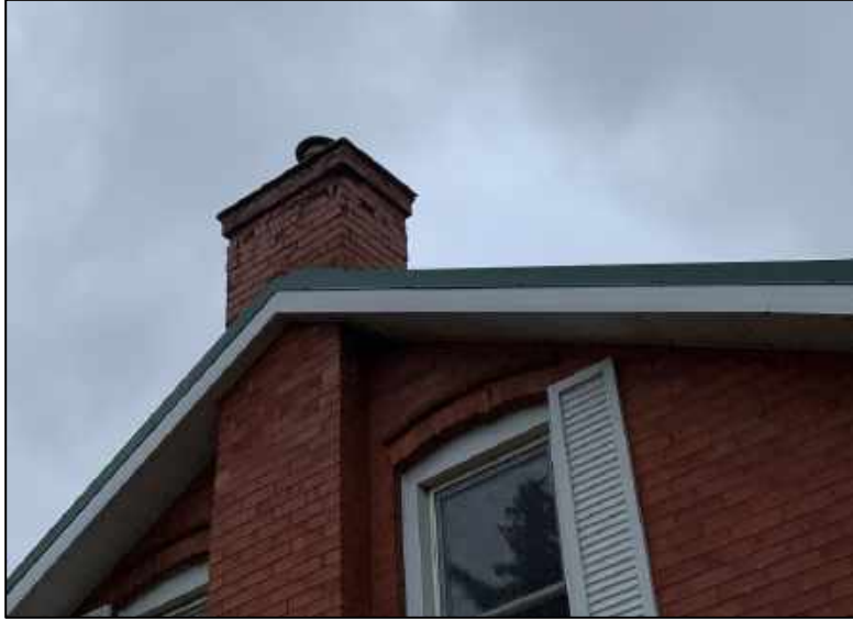
Photograph 14: Deterioration of chimney above roof line (west elevation).
