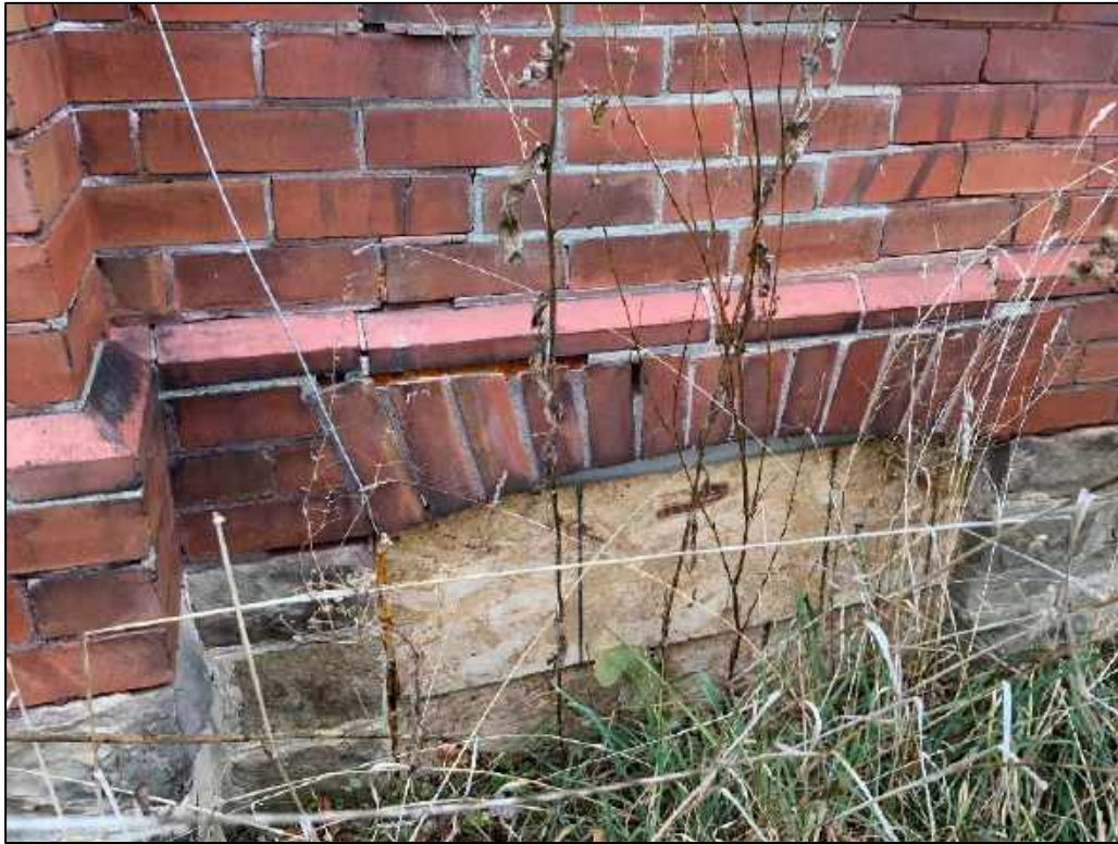
Photograph 16: Cracks and dropped brick above southernmost window (east elevation).
