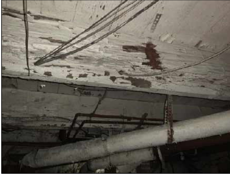
Photograph 5: Deteriorated and sistered joists.
