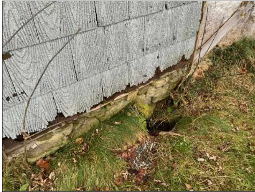
Photograph 22: Deteriorated wood shakes and hole against garage foundation.
