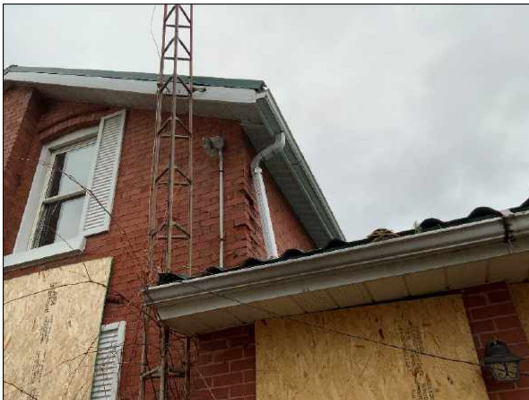
Photograph 17: Deteriorated brick above living room addition.
