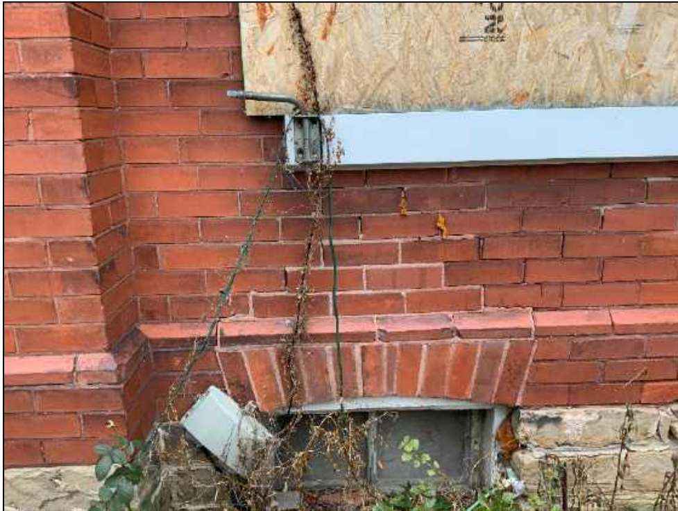
Photograph 12: Cracks in mortar joints above southernmost basement window (west elevation).
