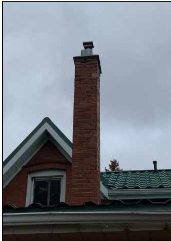
Photograph 19: Severe deterioration of brick at chimney above living room roof line.
