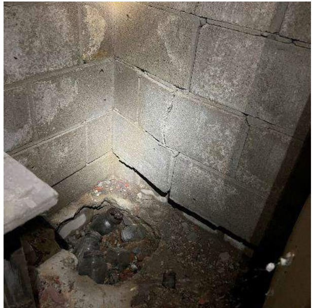
Buckling Concrete Block Foundation
