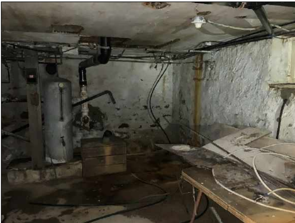
Photograph 8: Water ingress and staining.
