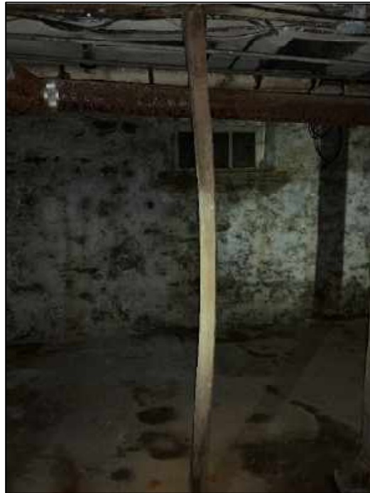
Photograph 6: Buckled prop in the intermediate bearing line.
