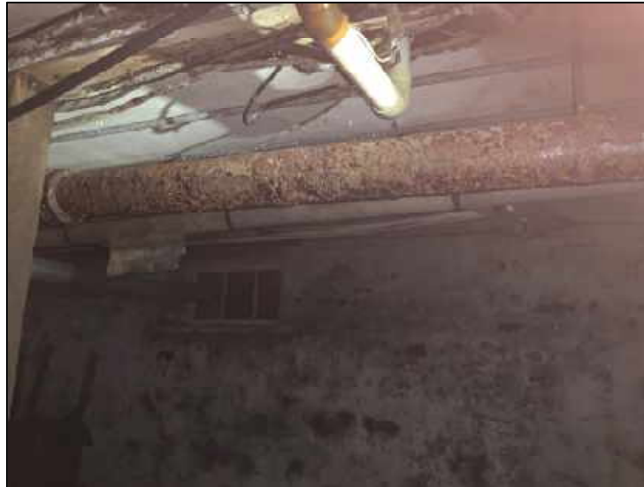
Photograph 9: Corrosion on exterior of steel pipe.
