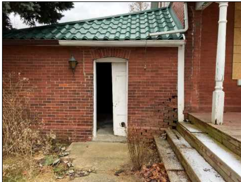
Photograph 23: Buckled and collapsed brick veneer on garage.
