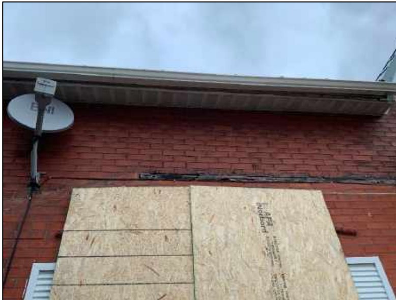
Photograph 15: Wood ledger with loose joints and diagonal cracks.
