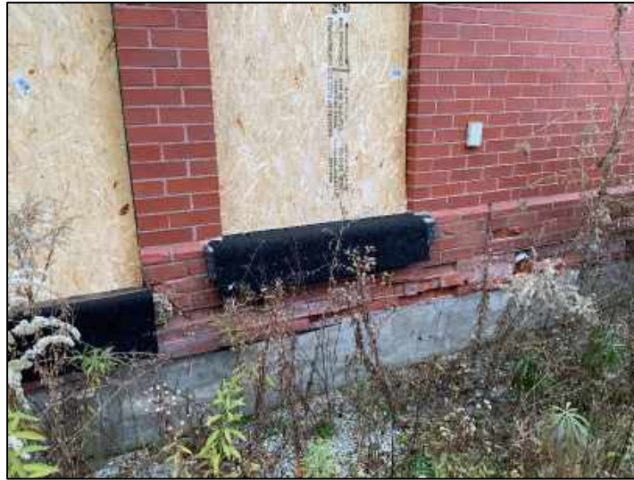
Photograph 18: Severe deterioration of brick below living room windows.
