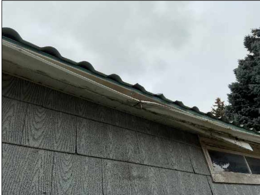
Photograph 21: Damaged eavestrough on garage.
