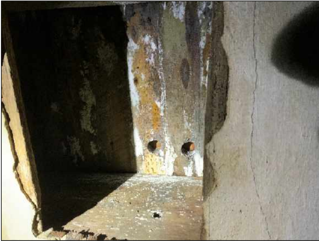
Photograph 7: Mold on floorboards/joists above.
