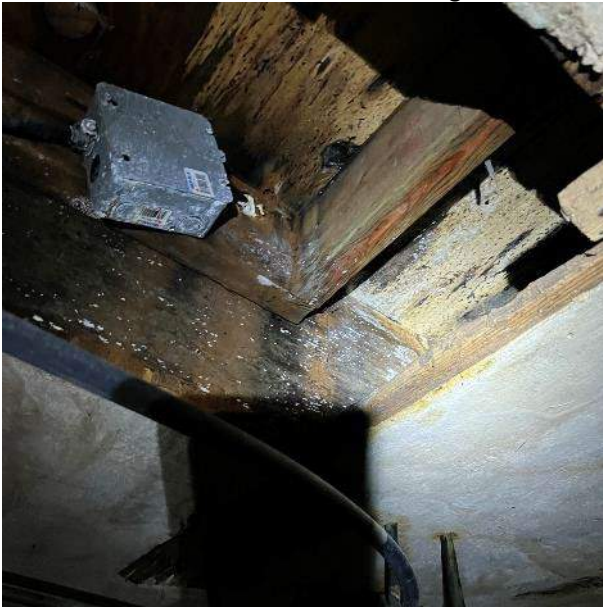
Basement Water Damage
