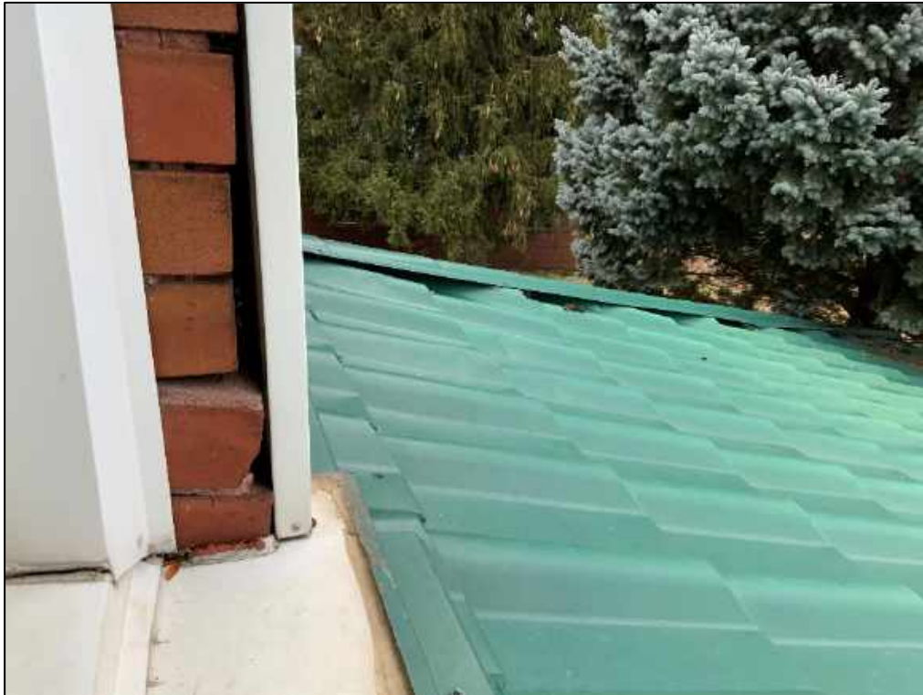
Photograph 20: Failed brick behind decorative shutter above garage.
