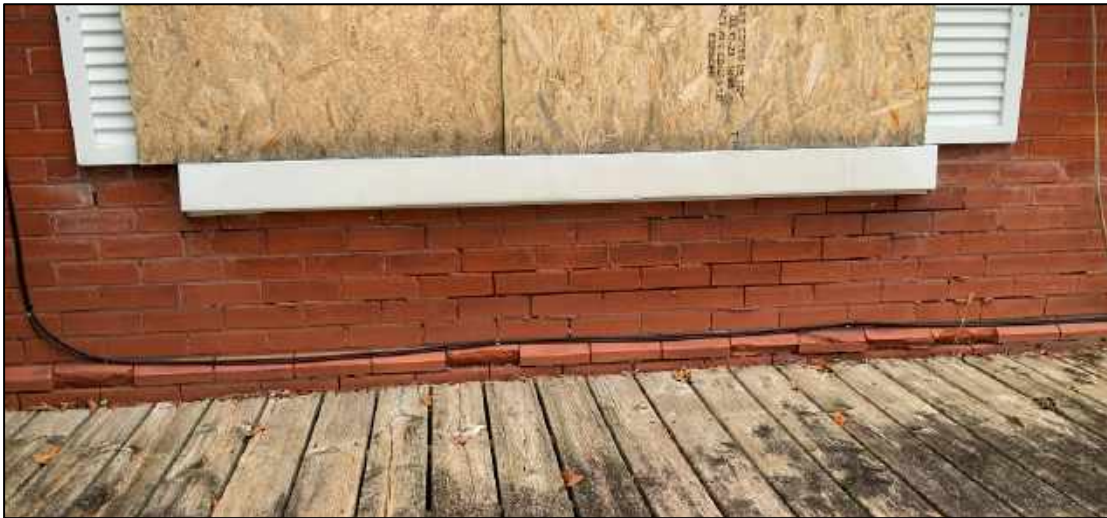
Photograph 11: General condition of exterior walls.
