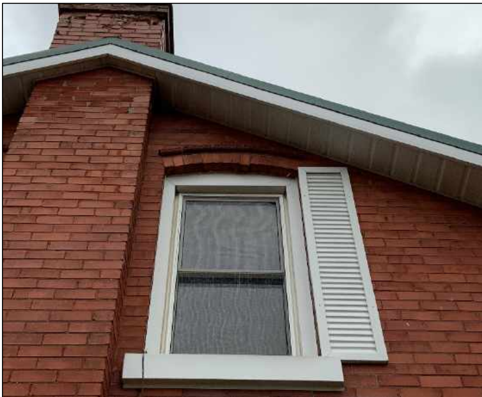
Photograph 13: Dropped brick above southernmost second-floor window (west elevation).
