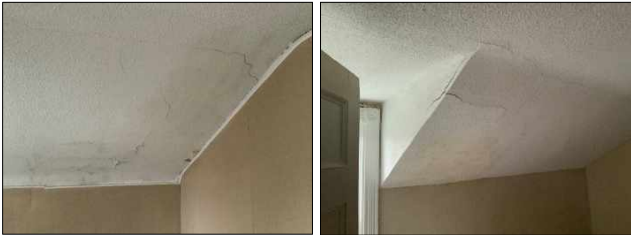
Photograph 2a & b: Cracks in north wing stair and adjacent bedroom.
