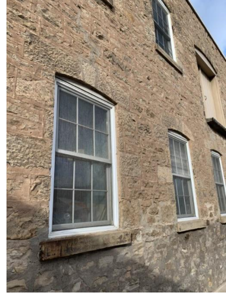
Figure 36: Evidence of parging and repair along the front elevation (Town of Halton Hills 2024)
