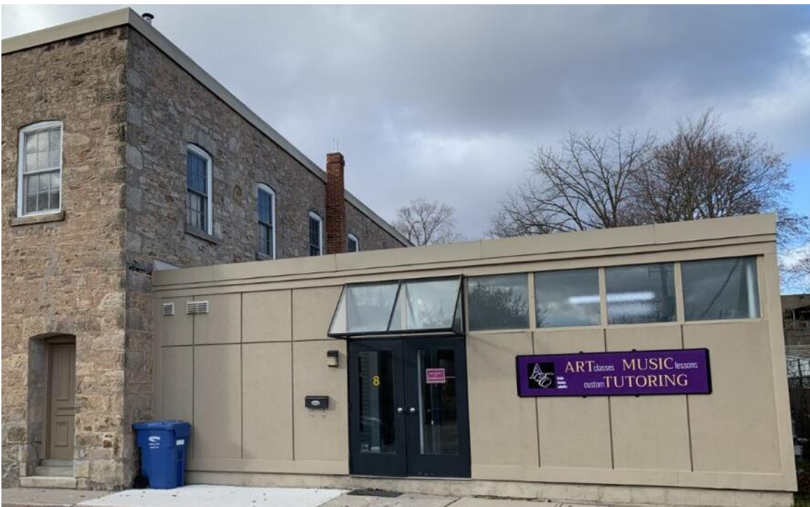
Figure 39: Partial side (northeast) elevation of the original building obscured by the one-storey concrete block addition (Town of Halton Hills 2023)
