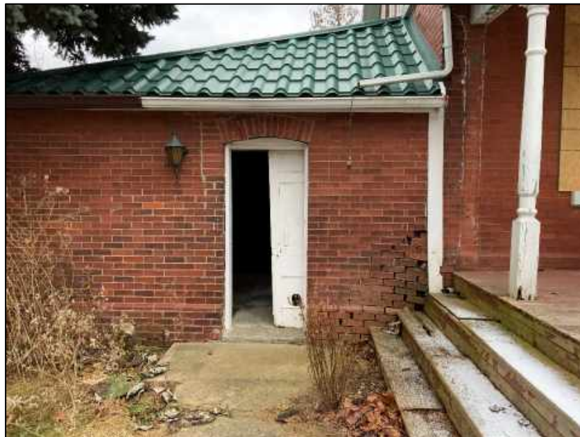
Photograph 23: Buckled and collapsed brick veneer on garage.
