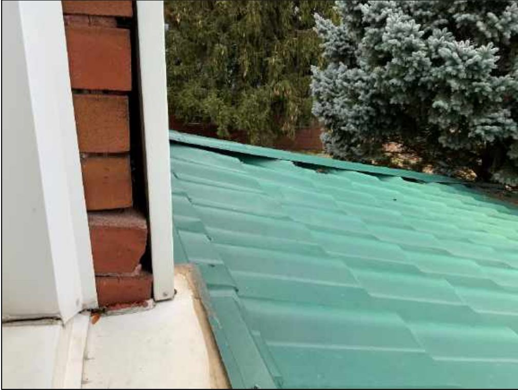
Photograph 20: Failed brick behind decorative shutter above garage.
