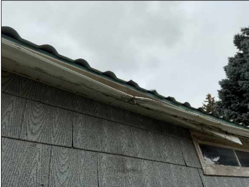
Photograph 21: Damaged eavestrough on garage.
