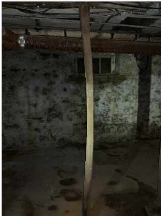
Photograph 6: Buckled prop in the intermediate bearing line.
