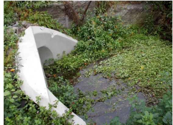
Photo 64: Station WQ8 Elmore Dr. storm outfall in wet weather, Sept. 22, 2021.
