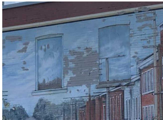
Figure 25: In-filled window openings at the upper storey, 26 Guelph Street (Town of Halton Hills 2023)
