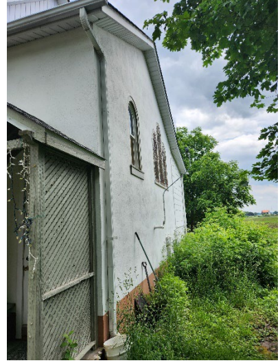
Figure 33: Rear (west) elevation of St. John's Anglican Church (Town of Halton Hills 2023)
