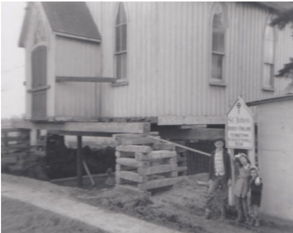
Figure 11: St. John's Anglican c.1958 during the basement construction (Courtesy of The Georgetown Vault)
