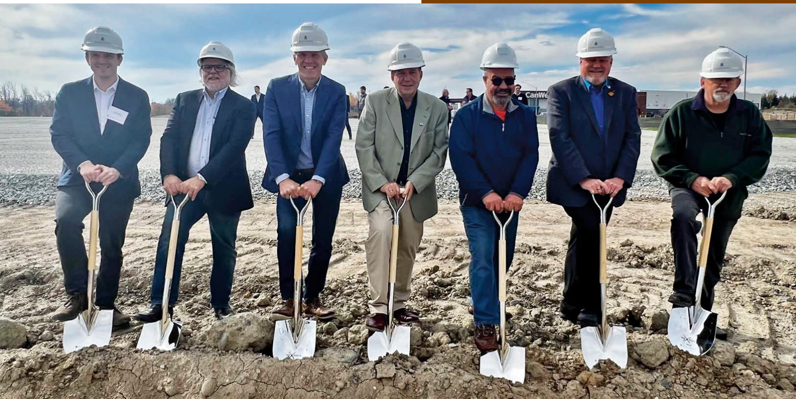
Panattoni Canada breaking ground on industrial building on Futura Drive in Halton Hills' Acton community
