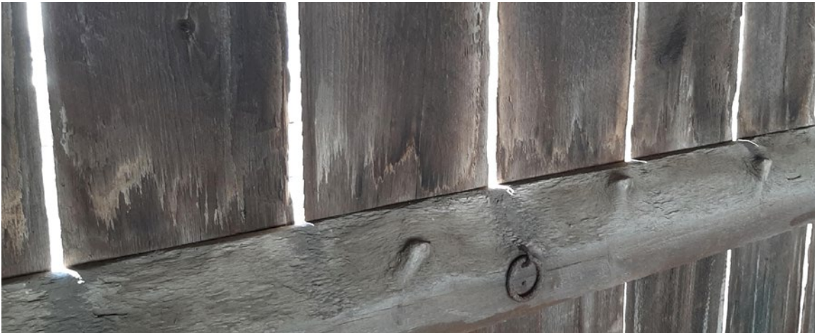
Figure 17: Horse damage and tie rings (Limestone Presbyterian Church 2022)
