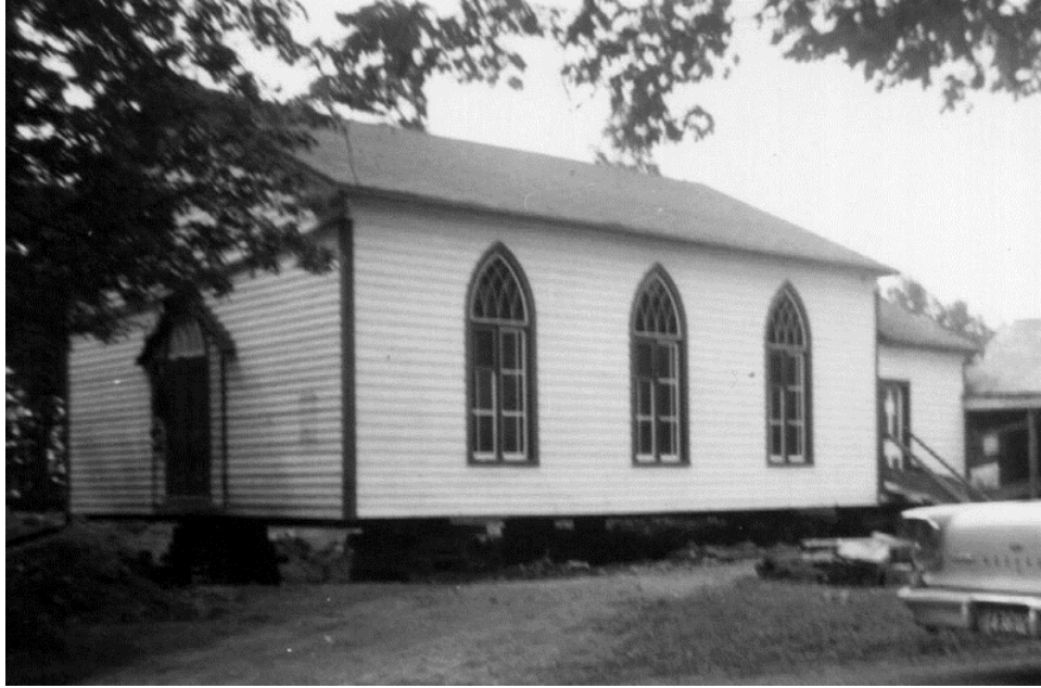
Figure 5: The church is raised on supports to dig out and construct the basement. The original doors remain in place inside the new front room (Brown 1961)
