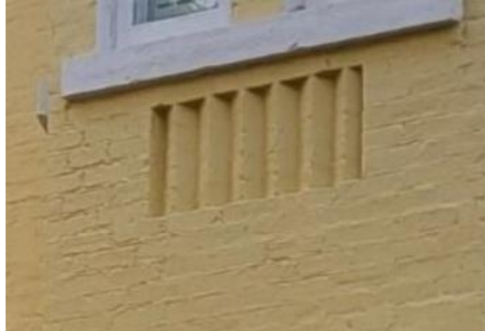
Figure 28: Inset "dogtooth" brick detailing on the projecting bay of 53 Charles Street (Town of Halton Hills 2024)
